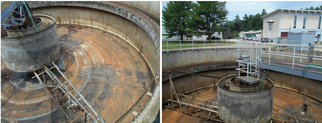
FIGURE 3-16 NITRIFICATION SETTLING TANKS
