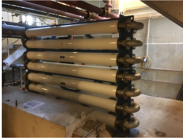
FIGURE 3-29 LARGE SLUDGE HEAT EXCHANGER
