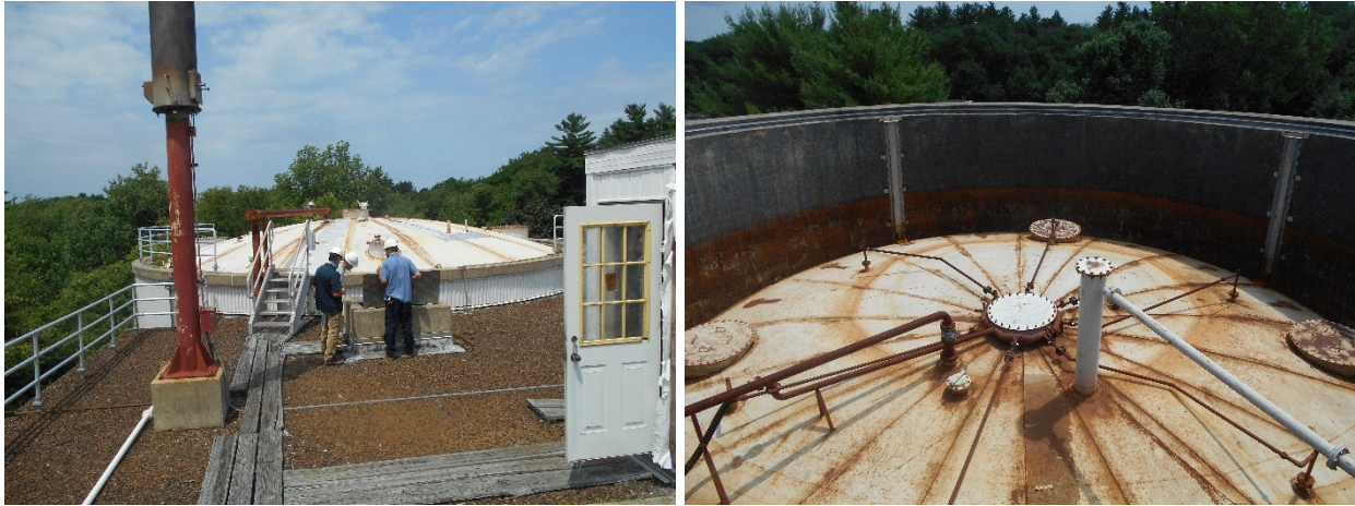
FIGURE 3-27 LARGE ANAEROBIC DIGESTERS
