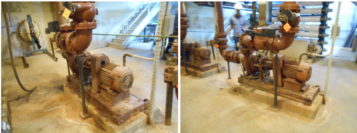
FIGURE 3-30 LARGE SLUDGE RECIRCULATION PUMPS
