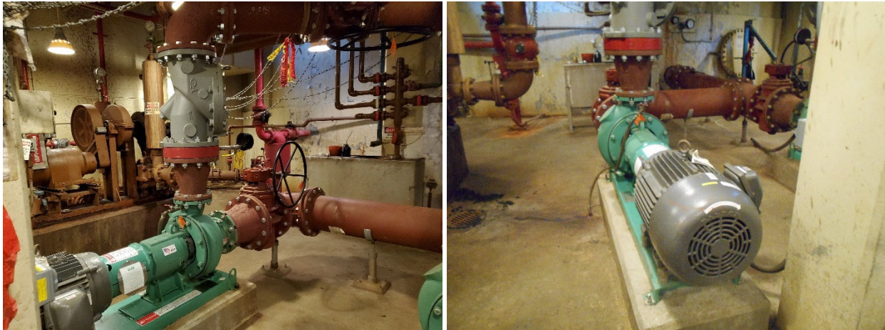
FIGURE 3-32 SLUDGE CHOPPER PUMPS
