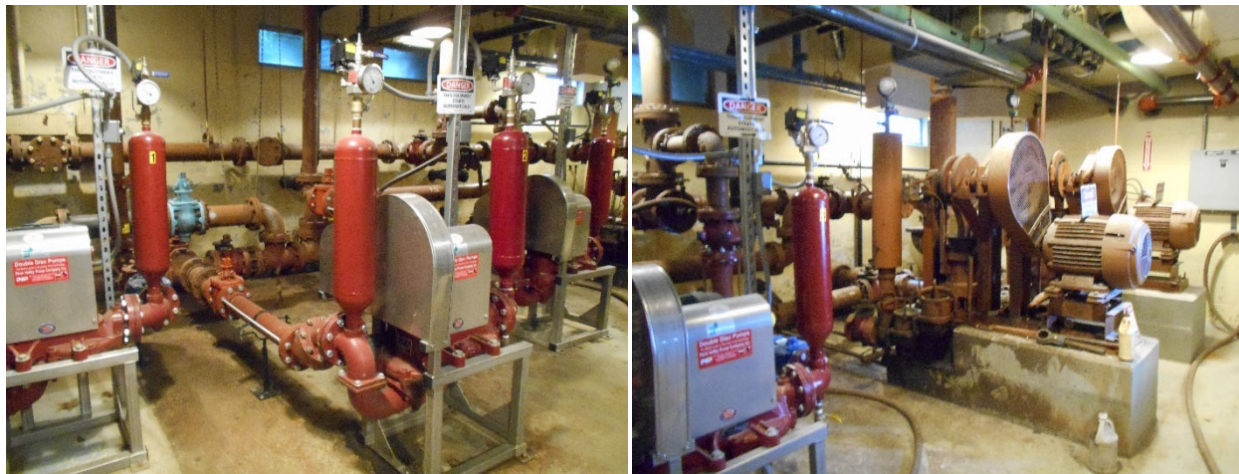
FIGURE 3-13 PRIMARY SLUDGE PUMPS
