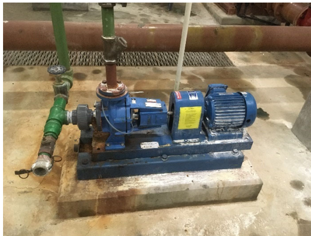
FIGURE 3-36 PLANT WATER PUMPS
