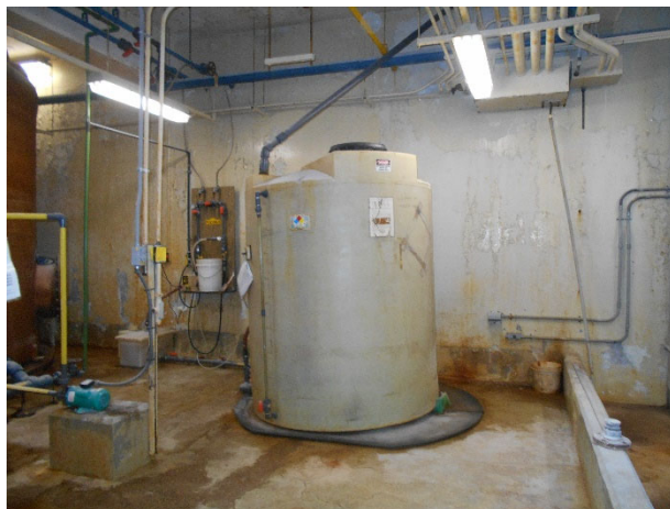
FIGURE 3-39 POLYMER STORAGE TANKS
