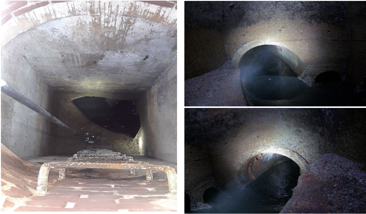
FIGURE 3-5 INFLUENT BYPASS MANHOLE
