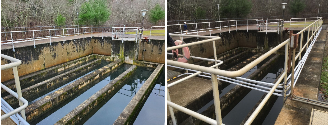
FIGURE 3-20 CHLORINE CONTACT TANKS
