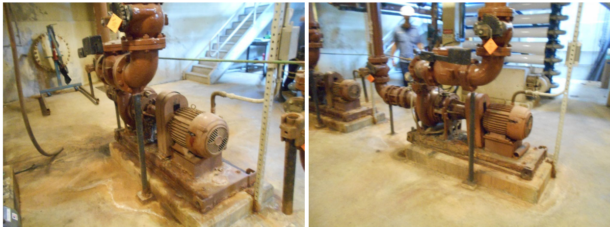
FIGURE 3-30 LARGE SLUDGE RECIRCULATION PUMPS
