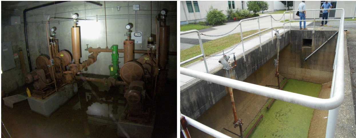
FIGURE 3-10 SEPTAGE HOLDING TANK AND PUMP STATION
