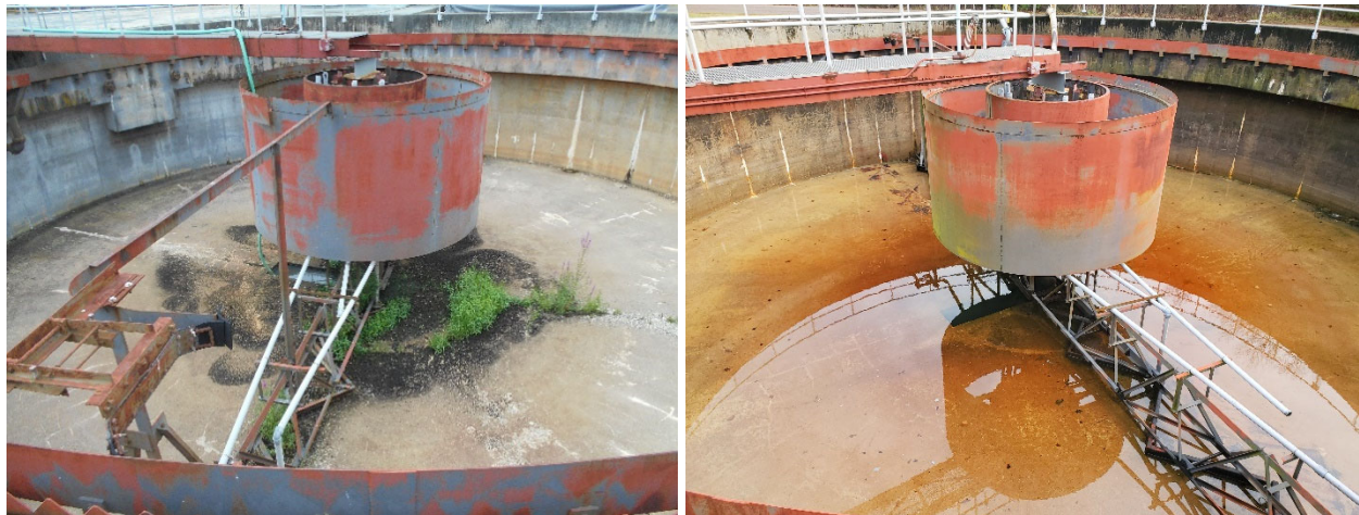
FIGURE 3-17 SECONDARY SETTLING TANKS
