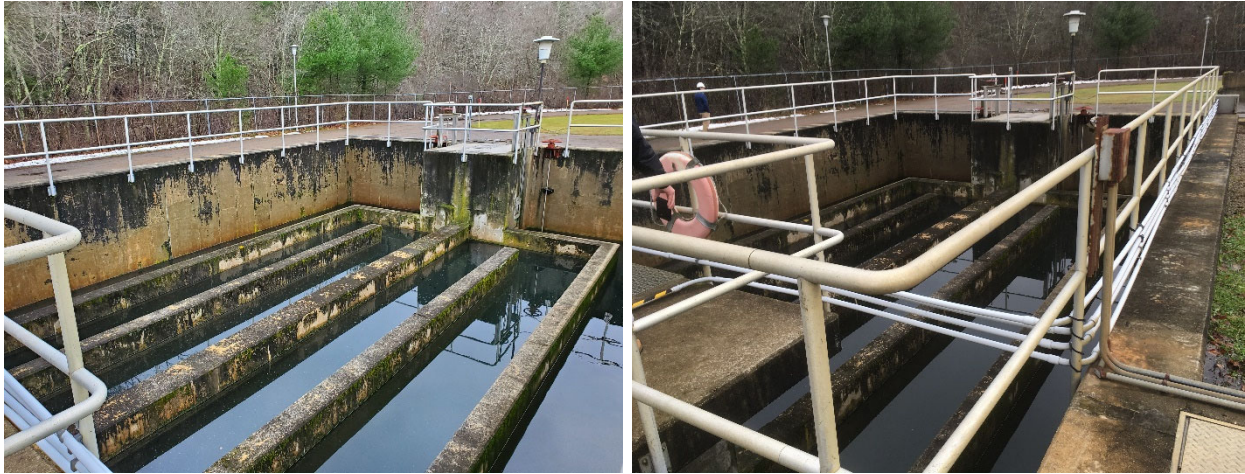
FIGURE 3-20 CHLORINE CONTACT TANKS
