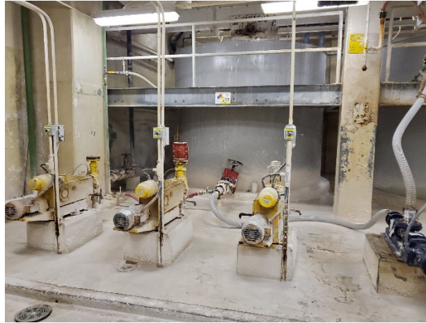
FIGURE 3-38 LIME SLURRY FEED PUMPS
