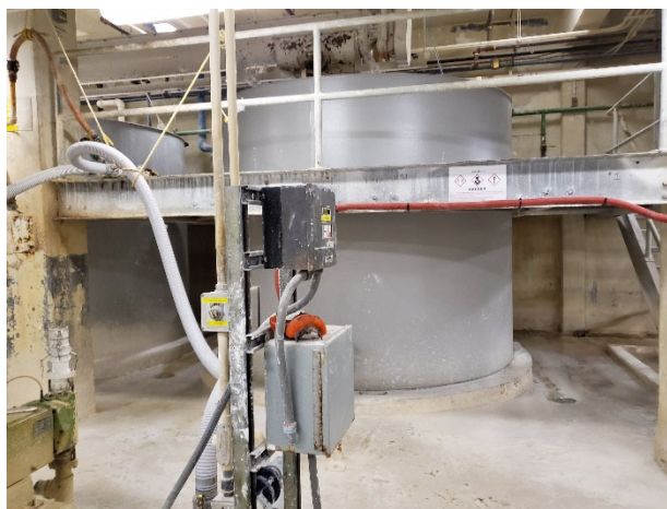
FIGURE 3-37 LIME SLURRY STORAGE TANKS
