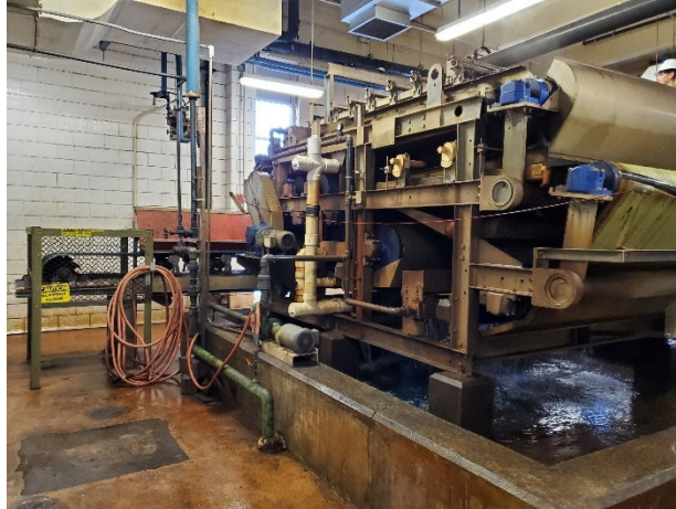
FIGURE 3-33 BELT FILTER PRESSES
