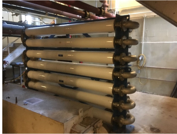
FIGURE 3-29 LARGE SLUDGE HEAT EXCHANGER
