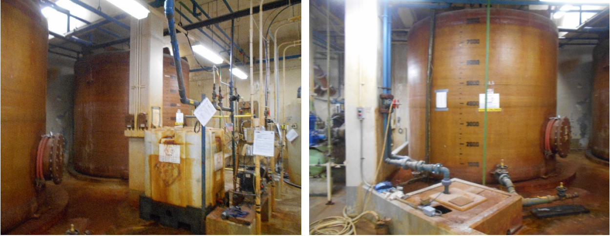
FIGURE 3-9 FERRIC CHLORIDE TANKS
