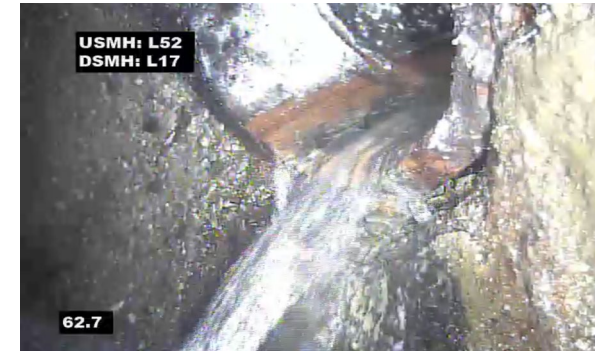
Infiltration @ Joint: Approx. 5760 GPD
