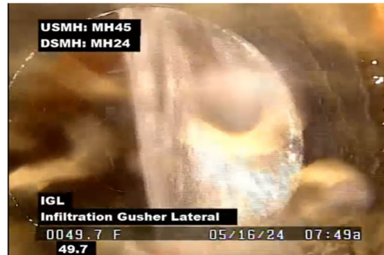
Infiltration @ Joint: Approx. 28,800 GPD
