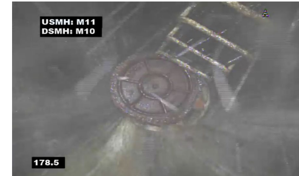
Infiltration/Inflow @ Manhole Cover
