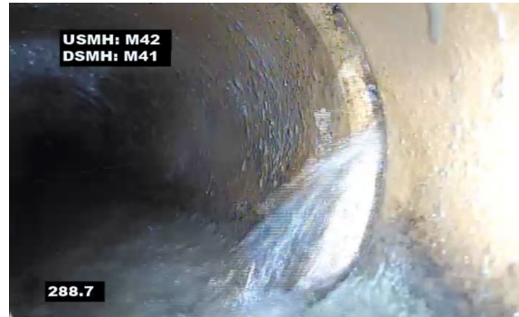
Infiltration @ Joint: Approx. 7200 GPD
