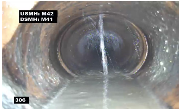
Infiltration @ Joint: Approx. 7200 GPD
