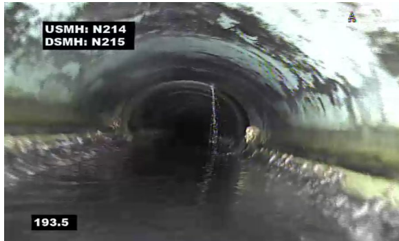
Infiltration @ Joint: Approx. 1440 GPD
